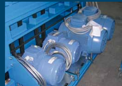
Motors in dry zone
